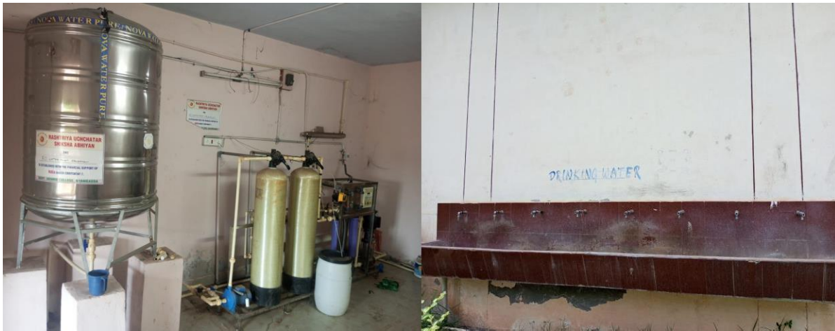
RO plant drinking water for students
