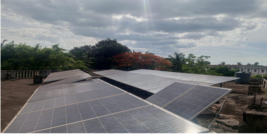
Solar Panels on the Rooftop of main Building
