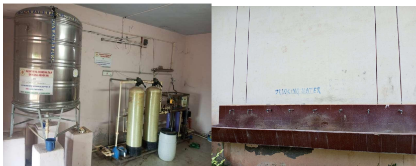
RO plant drinking water for students
